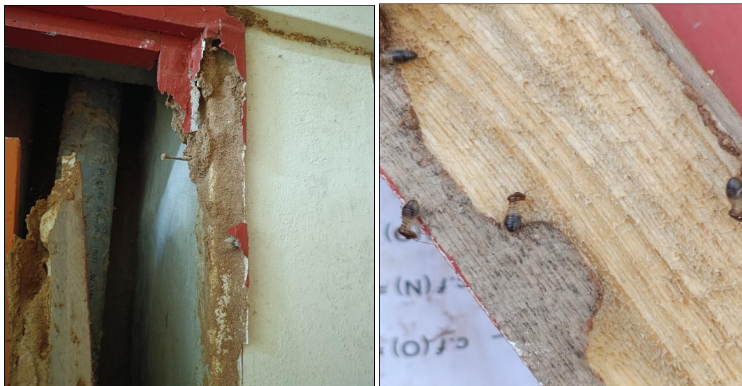
Fig 2: Damage caused by termites
