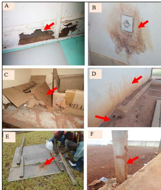
Fig 6: Termite damage on buildings A: ceiling, B: Electrical outlet, C: storage carton, D: wall of a building, E: bulletin board, F: Hangar support.
